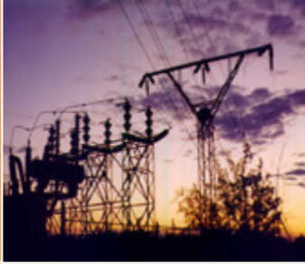
Frank Channel substation (servicing Rae/Edzo) at midnight.
