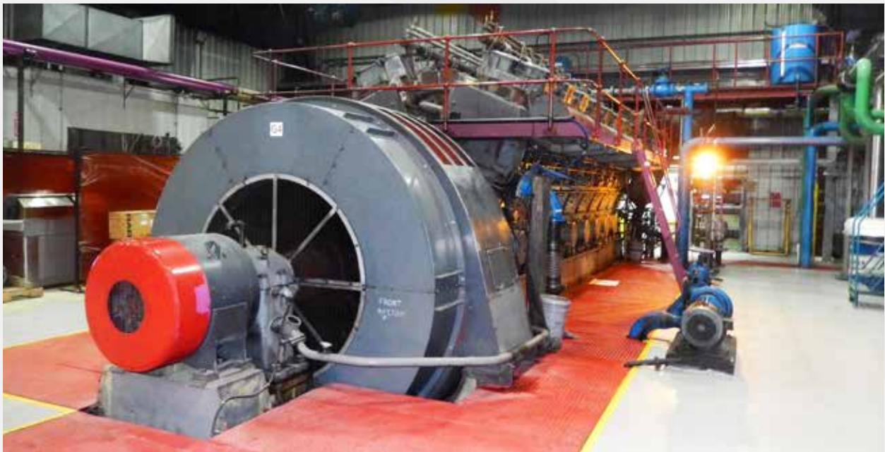
Diesel generators provide back up power to hydro communities to ensure reliability of service.
