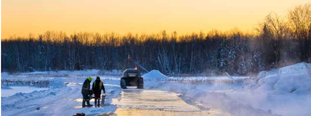
In 2019-20, NTPC constructed the Taltson Winter Road for the first time in many years. The road is needed to bring in equipment prior to the upcoming refurbishment.
