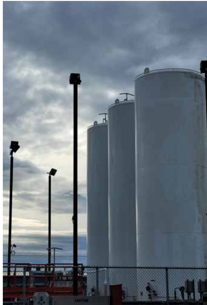
In the fall of 2022, a third storage tank for LNG was installed in Inuvik, helping to reduce diesel usage and greenhouse gas emissions.
