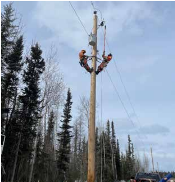
The arrival of new housing units in Jean Marie River required installation of new power poles and the replacement of the transformer substation. This major project was completed in fewer hours than budgeted because of great teamwork and widespread community cooperation and support
